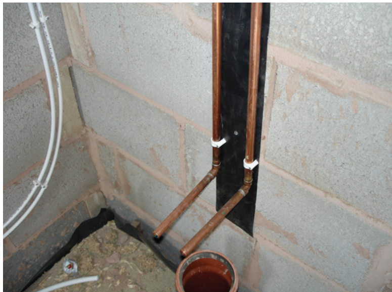
Figure 1.1 Examples of typical plumbing materials. Hot and cold feed in copper to the right, plastic heating pipes to the left, and plastic drain connection below copper pipes
