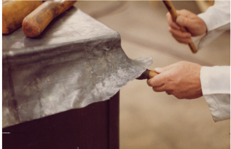
Figure 4.19 Sheet lead work (Reproduced with the kind permission of the Lead Sheet Association)
