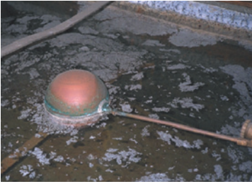
Figure 4.9 Galvanised tank corrosion
