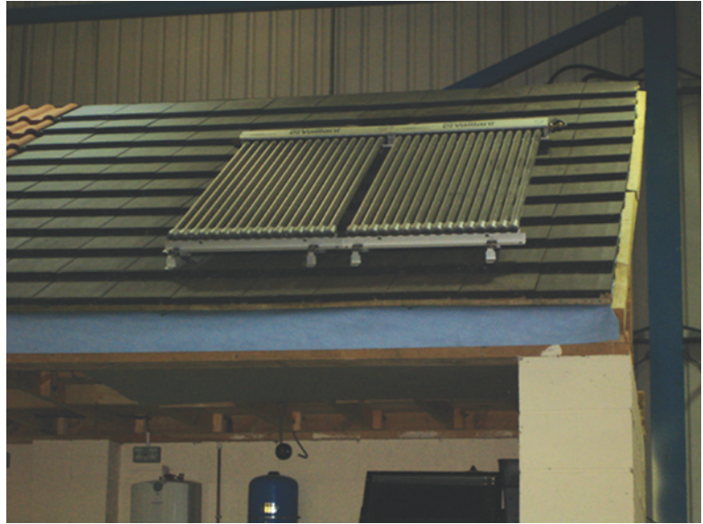
Figure 11.2 Example of a solar panel installation in a plumbing workshop
